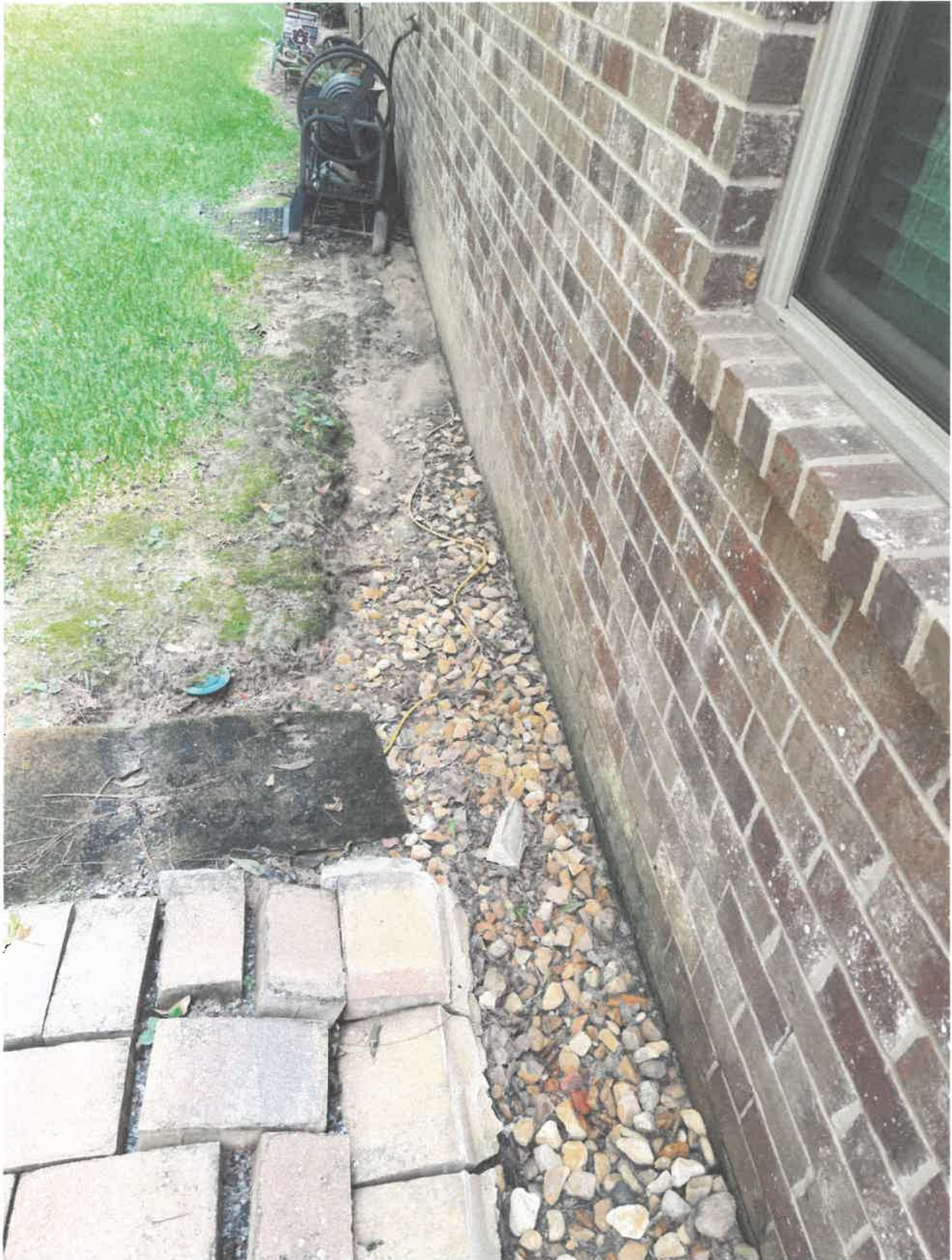
Erosion and sand deposits on west side of house.
