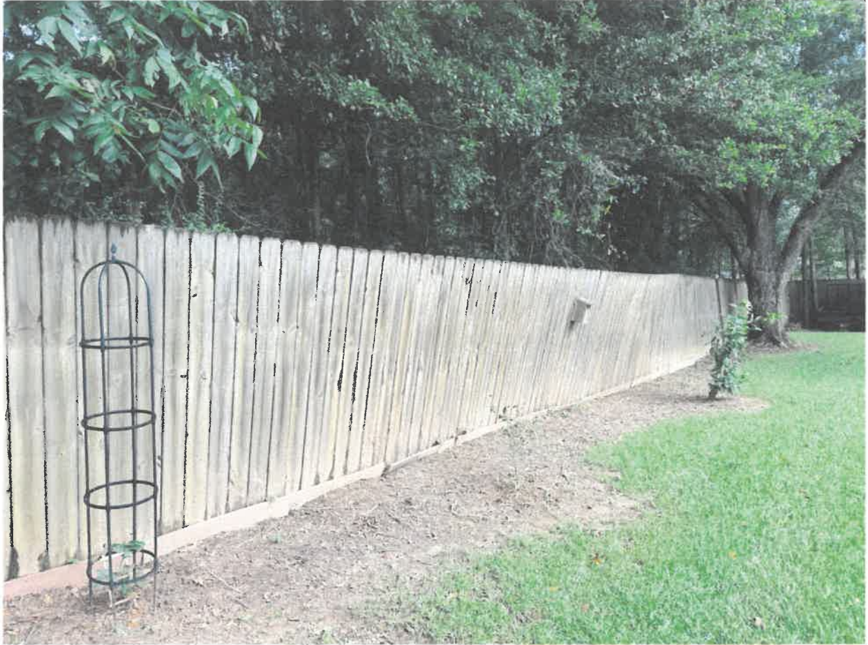
Water saturation continues to undermine the fence causing the fence to lean.
