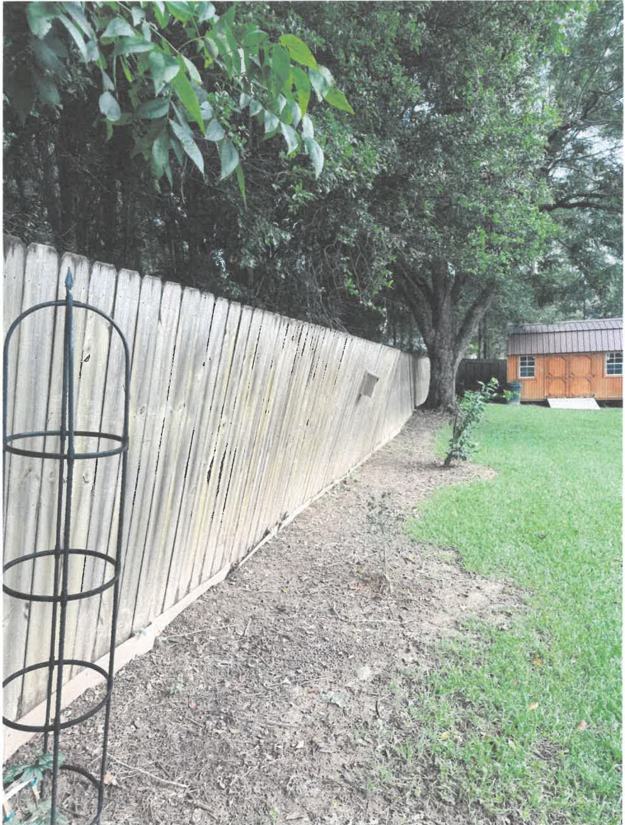
Water saturation continues to undermine the fence causing the fence to lean.
