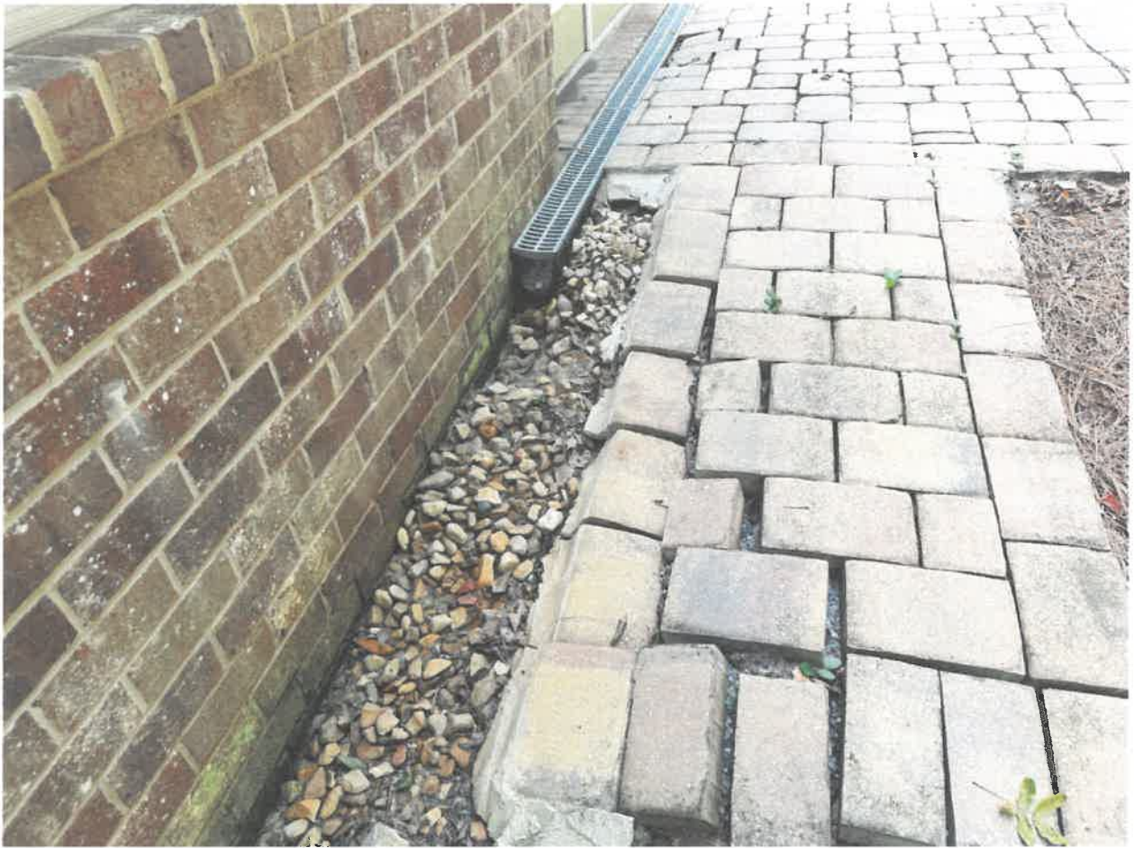
Erosion on west side of house.
