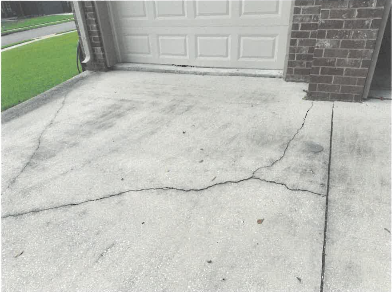
Cracking of driveway due to erosion.
