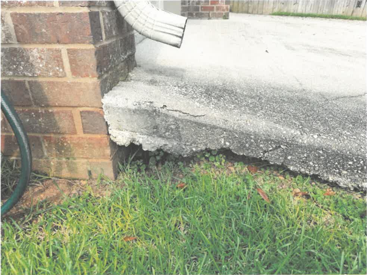
Gap underneath driveway due to erosion.
