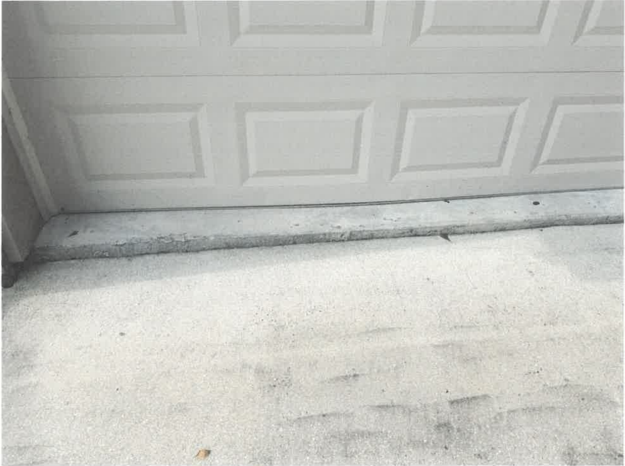
Drive has dropped about 2-3 inches due to water undermining.
