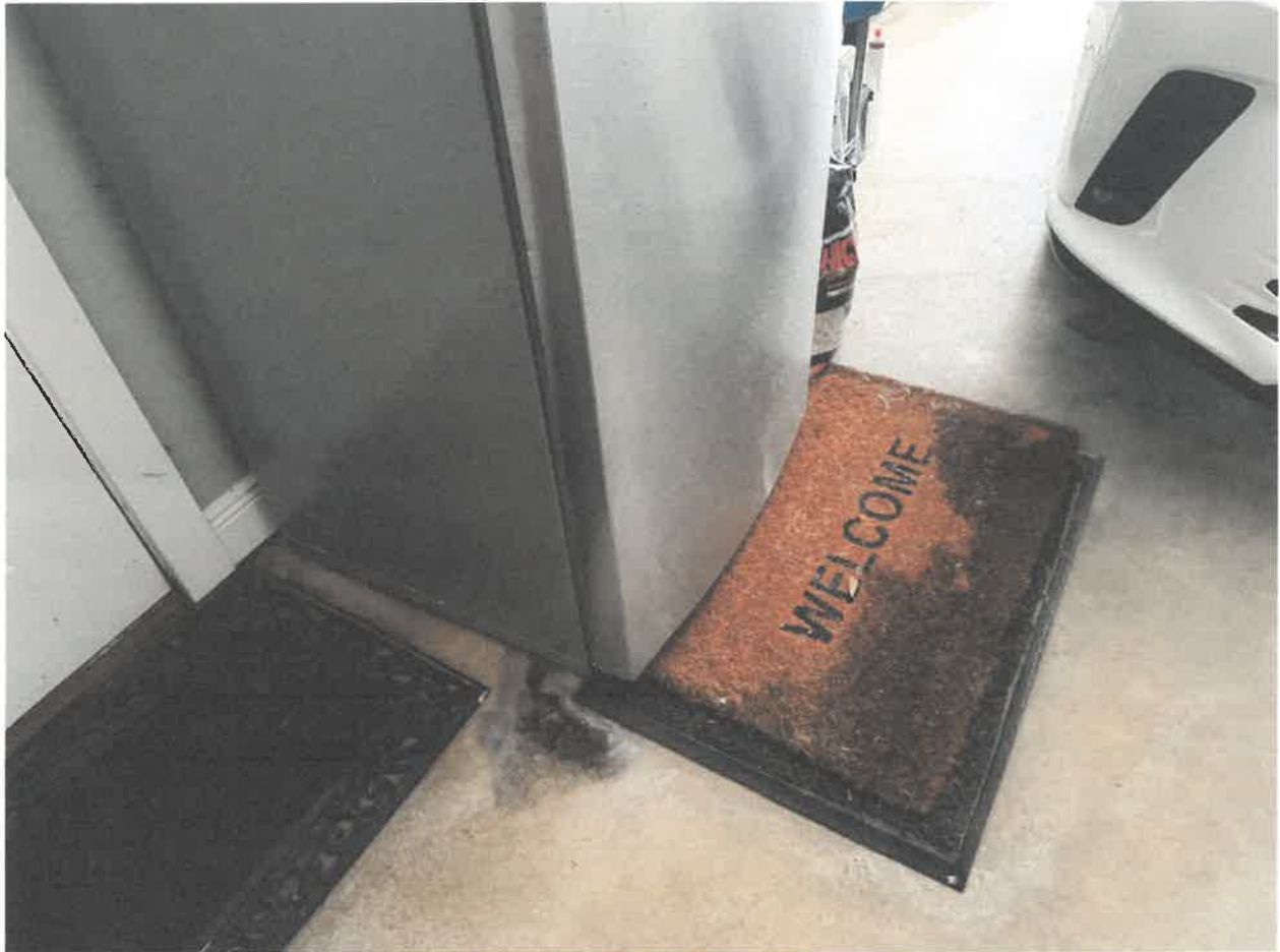
Water getting into garage due to sand deposits redirecting waterflow along the west side of the house.
