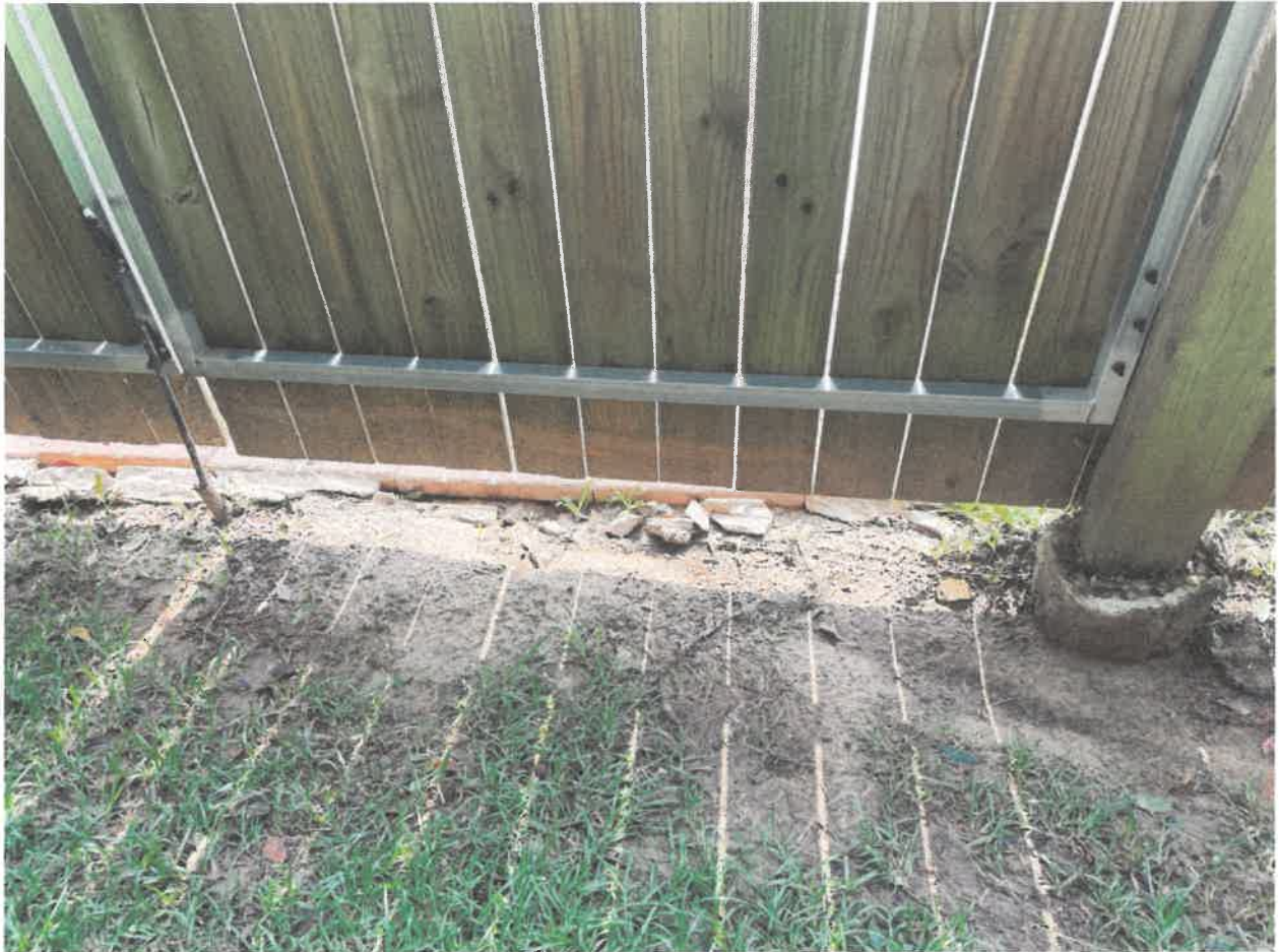
Erosion west of driveway pad.
