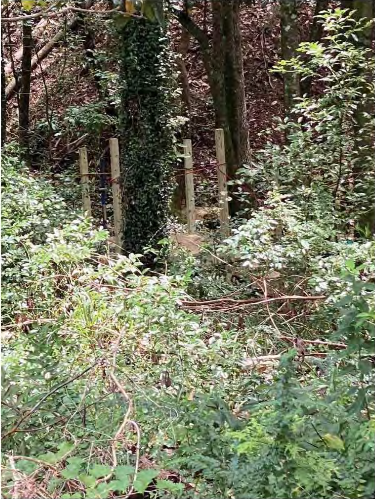
UNPERMITTED STAIRS UNDER CONSTRUCTION
